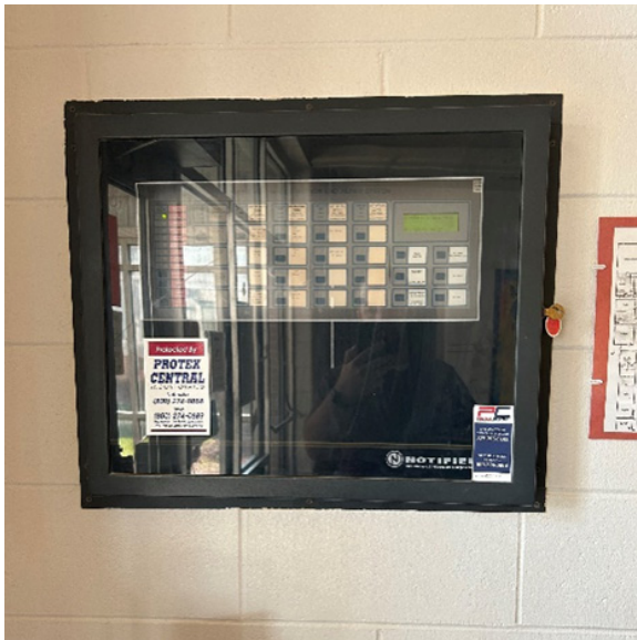
Fig. 3.6.9: Fire Alarm Control Panel, 2023.
