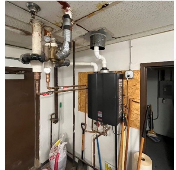
Fig. 3.5.4: Domestic Hot Water Heater, 2023.
