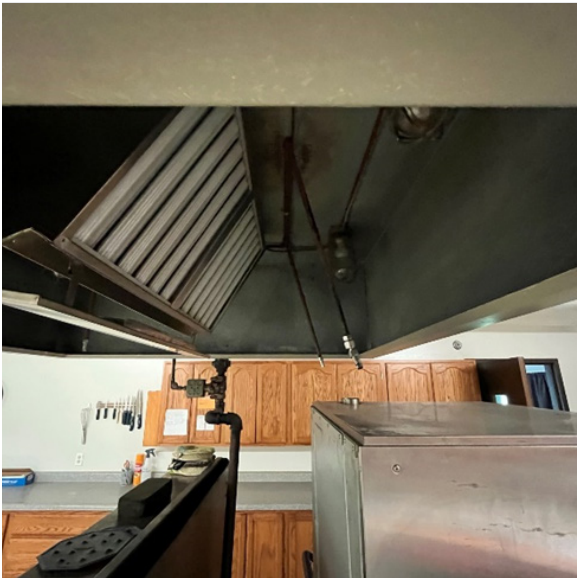
Fig. 3.5.9: Kitchen Hood Doesn't Extend Over Combi. Oven, 2023.
