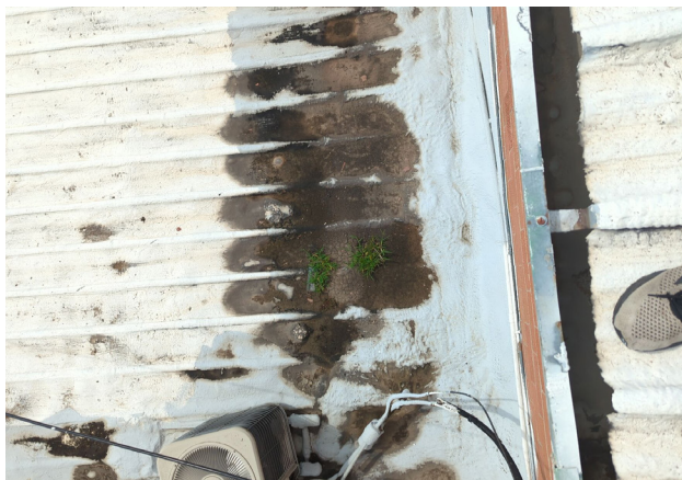
Fig. 3.4.42: Water build up, 2023.
