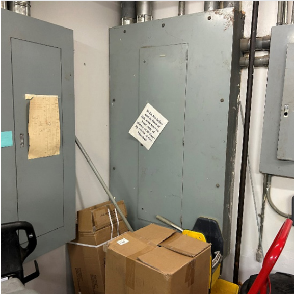
Fig. 3.6.4: Main Panelboard and Branch Panelboards, 2023.
