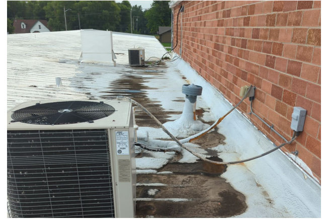
Fig. 3.4.38: Water build up, 2023.
