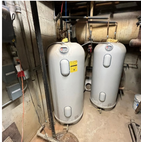
Fig. 3.5.14: 1961 Original Building: Domestic Hot Water Heaters, 2023.
