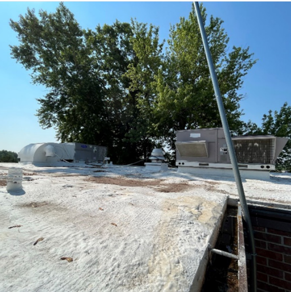
Fig. 3.5.7: Lunch Room & Kitchen Rooftop Units, 2023.
