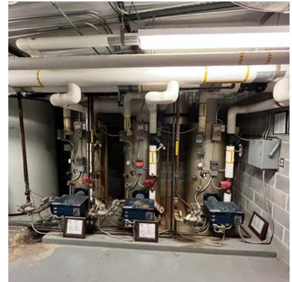
Fig. 3.5.22: 1994 Addition: Hydronic Hot Water Boilers, 2023.
