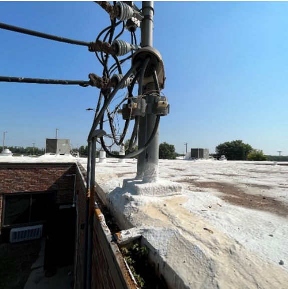
Fig. 3.5.10: East & West Wing Rooftop Units, 2023.
