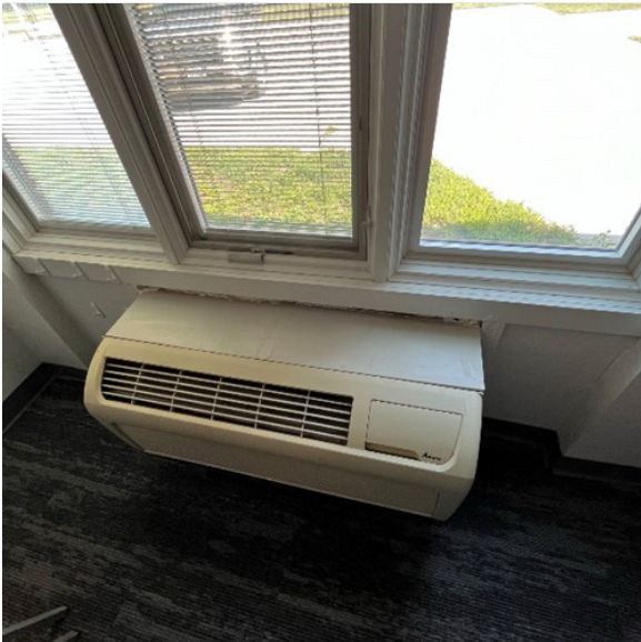
Fig. 3.5.8: Packaged Terminal Air Conditioner (PTAC), 2023.
