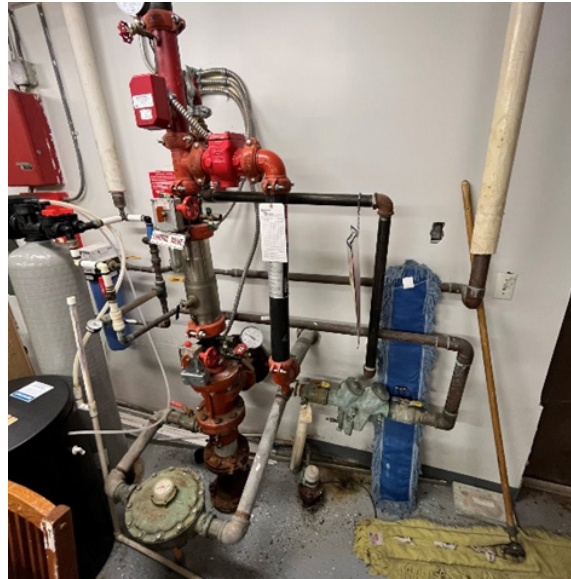
Fig. 3.5.3: Combination Fire/Water Service Entrance, 2023.
