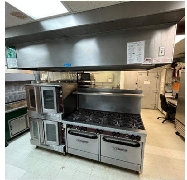
Fig. 3.5.20: Type 1 Kitchen Grease Hood, 2023.
