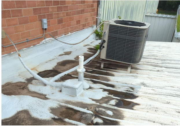
Fig. 3.4.37: Water build up, 2023.
