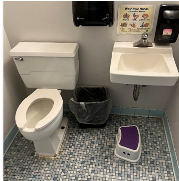
Fig. 3.5.5: Typical Restroom Plumbing Fixture, 2023.
