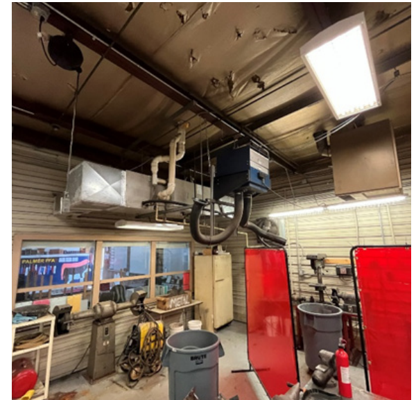
Fig. 3.5.19: Shop: Ag Classroom Split System A/C & Shop Unit Heater, 2023.
