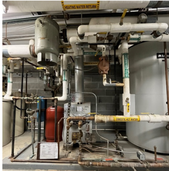
Fig. 3.5.12: 1994 Addition: Domestic Hot Water Heater & Storage Tank, 2023.
