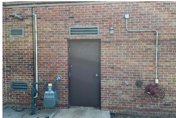
Fig. 3.5.1: Natural Gas Service, 2023.
