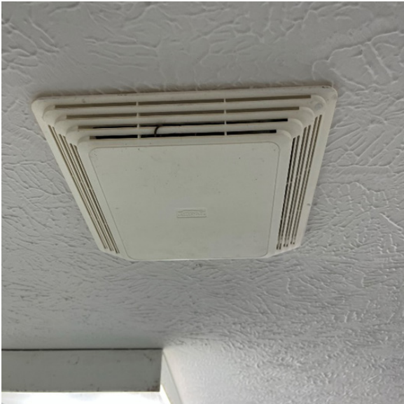
Fig. 3.5.11: Typical Ceiling Mounted Exhaust Fan, 2023.
