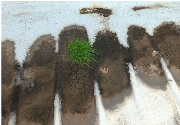
Fig. 3.4.40: Water build up, 2023.
