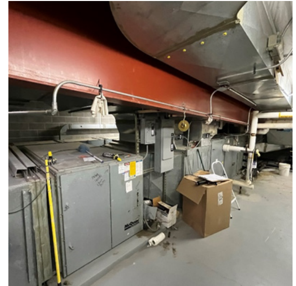
Fig. 3.5.17: 1994 Addition: Multi-Zone Air Handling Unit, 2023.
