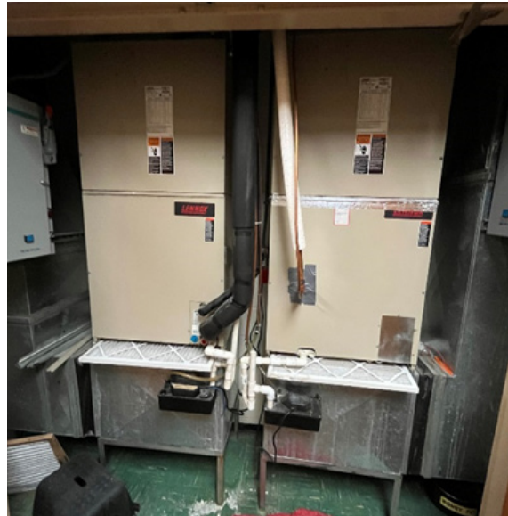
Fig. 3.5.16: Typical Split System Indoor Units, 2023.
