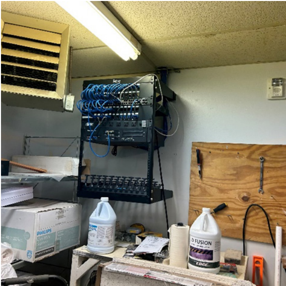
Fig. 3.6.5: Main Telecom Equipment Rack, 2023.
