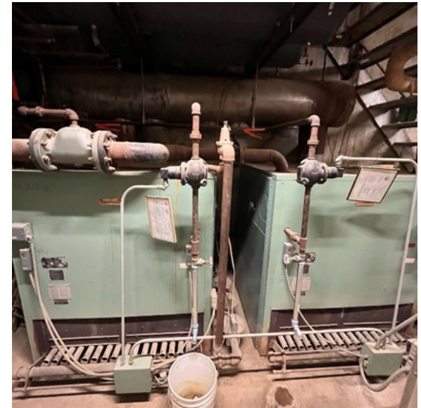
Fig. 3.5.21: 1961 Original Building: Hydronic Hot Water Boilers, 2023.
