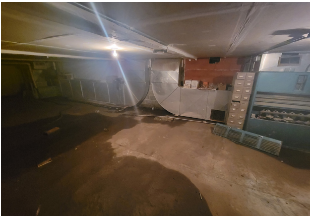
Fig. 3.2.3: Mechanical Lower Level, 2023.
