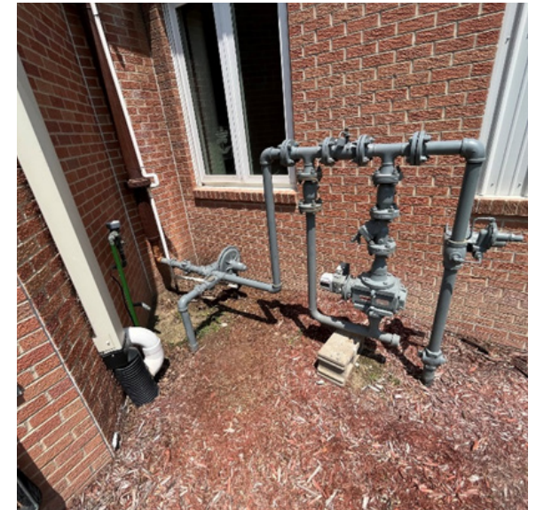
Fig. 3.5.15: Natural Gas Service, 2023.
